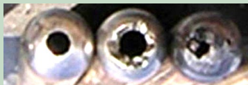
Push Rods which are inside the Push Rod tubes, moving up and down
